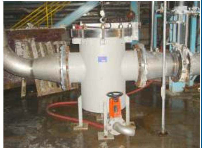
Industrial Liquid Trap Installed
